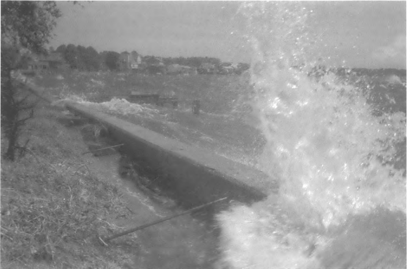
Water pours over a bulkhead in the Colington Harbour subdivision of Kill Devil Hills during a storm. These waves are from the Roanoke Sound, not the open sea, and have taken a toll on the land that used to support this seawall.
