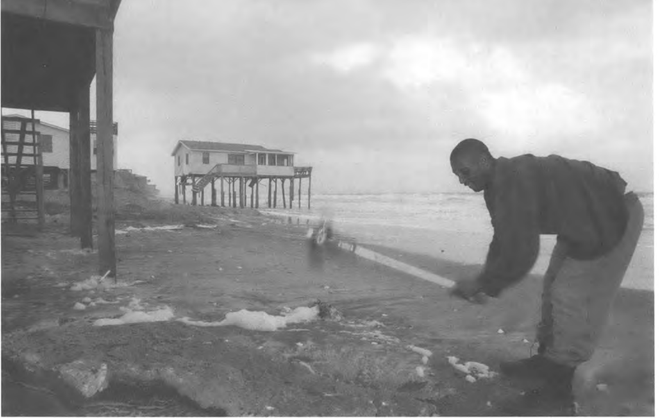
Above: A worker uses a sledgehammer to break up concrete from a damaged driveway in Nags Head after a storm.
