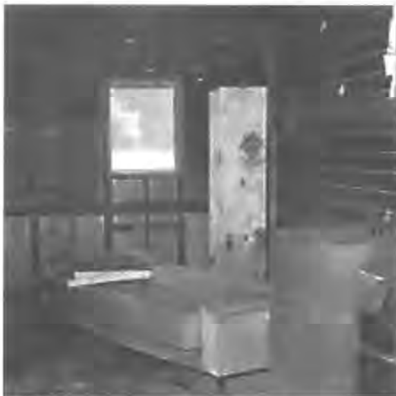
Migrant farmworkers endure cramped, ramshackle quarters with inadequate heating, lighting, and plumbing. Photo courtesy of NC Legal Aid.
