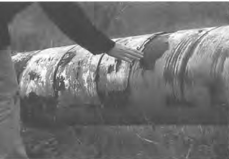
Section of pipe over Marble Creek in Southeast Austin. This pipe was actually replaced with new pipe. Photo courtesy of Stefan Wray.
